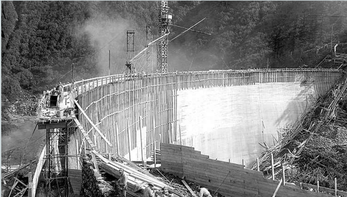
Salmon Creek Dam Under Construction ~ 1913. 1 st constant angle variable radius dam in world.
