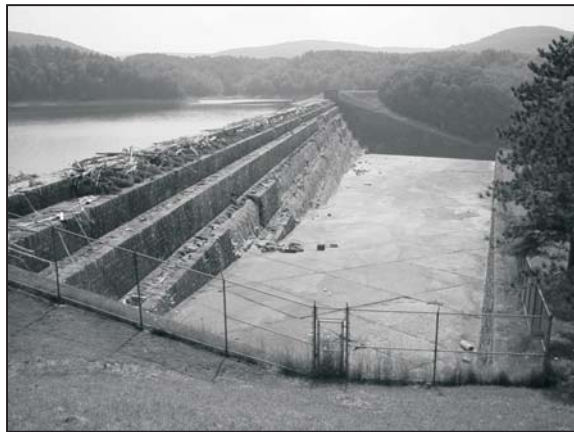
Figure 1. View of existing spillway as of 2004 (note dislodged facing stones).
